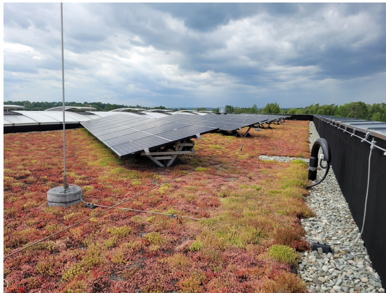
Bio-solar roof (Cracow)
