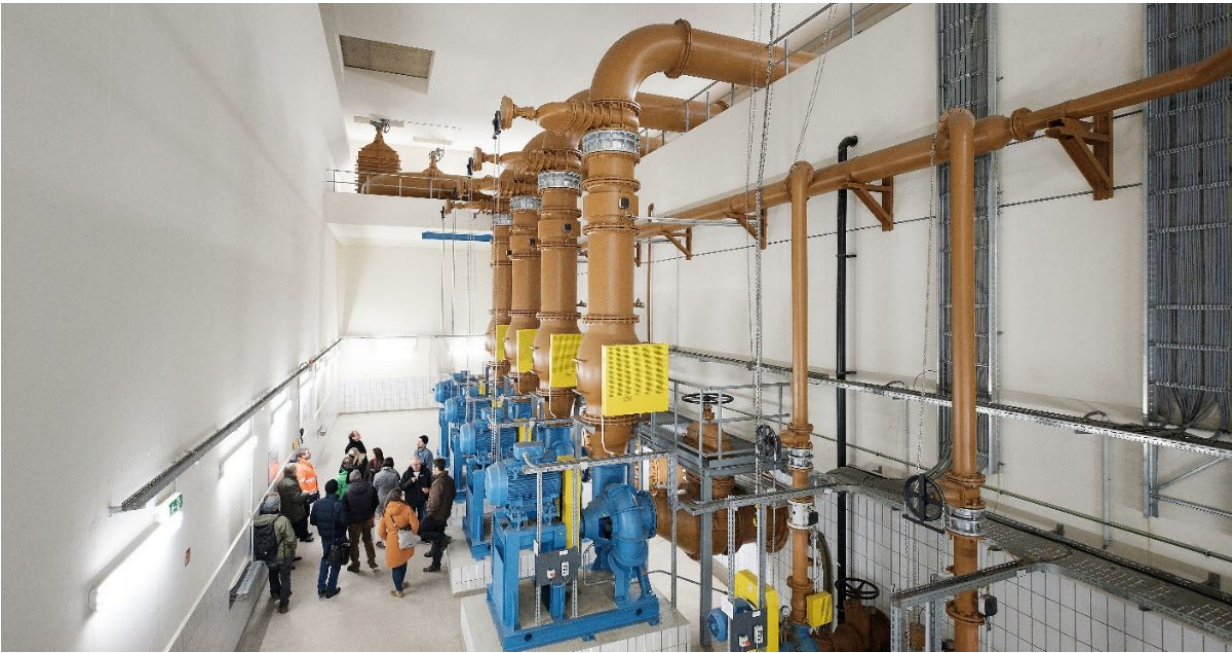
Inside a pumping station in Cologne: insights into the urban drainage strategy in Cologne city centre.
