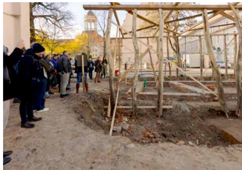
Participants visited the construction site of a pavilion which is being built with organic and recycled materials.
