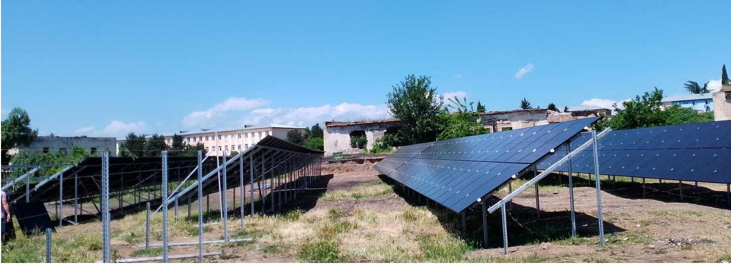
Some of the solar panel rows in Eredvi Municipality
